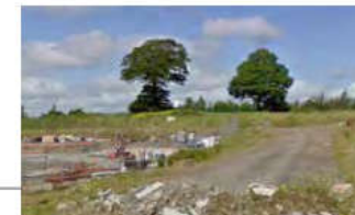
View of former site access road adjacent Neighbourhood Centre Site and beyond to two existing trees on site (tree visible to the right to be retained)
